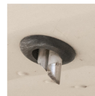
Heater Fuel Drains
