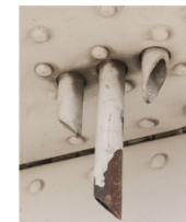
Battery Vents & Batter Drains
