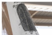
Fresh Air Inlet
