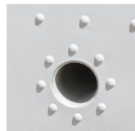
Heater Combustion Blower Intake
